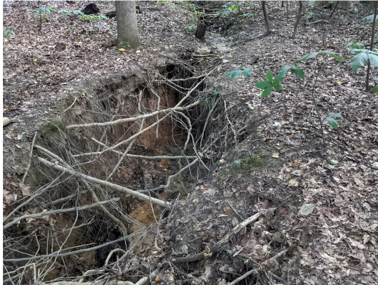
Site 1, Photo 3: Start of large erosion downstream of failed culvert (Looking Upstream (East))
