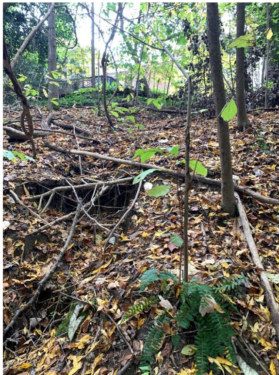
Site 4, Photo 12: Slope Erosion behind 102 Montague Circle
