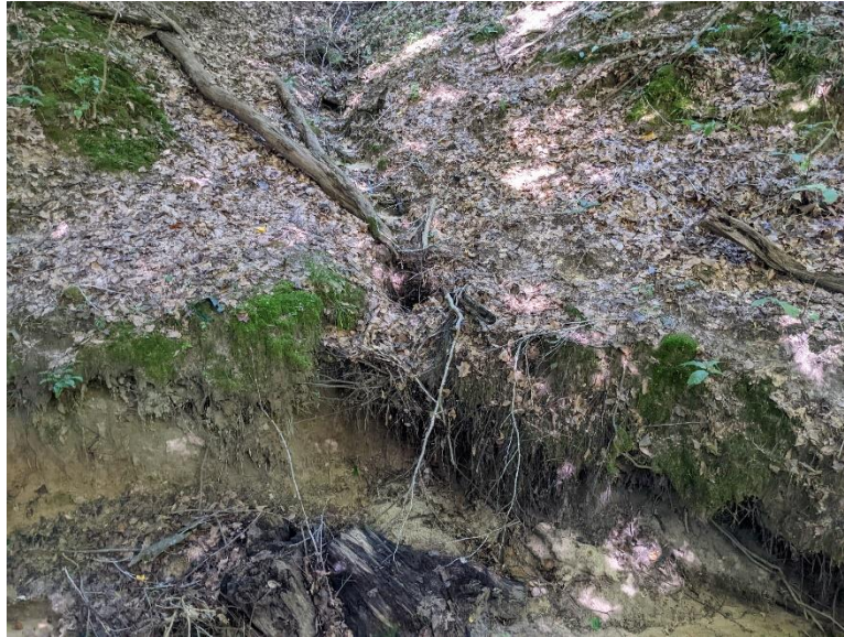
Site 4, Photo 7: Slope Erosion behind 266 East Queens Drive (Tie-in to Primary Stream, Looking North)
