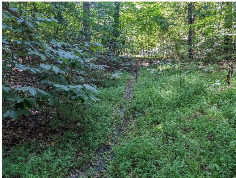
Site 4, Photo 2: Existing Geotextile Lined Channel Continues into the Woods (Looking Downstream (East))
