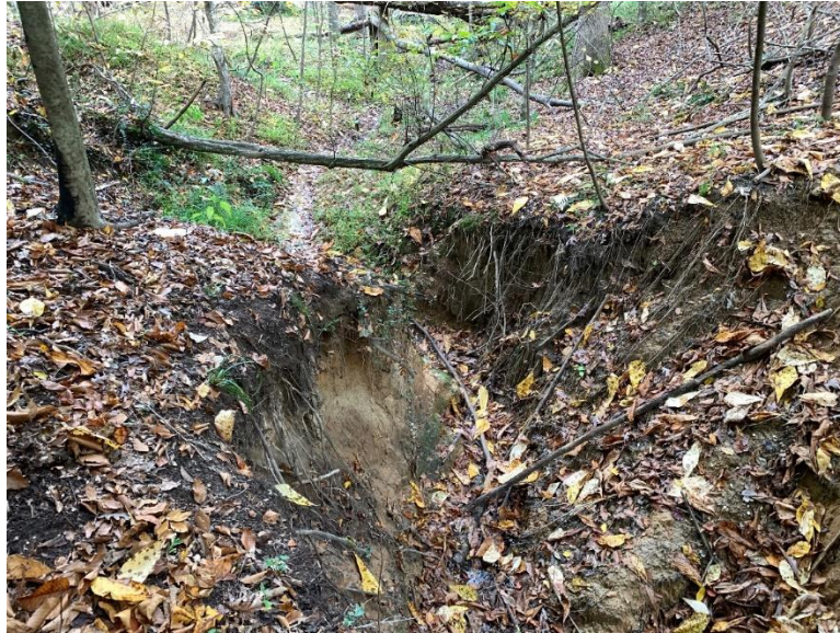
Site 8, Photo 7: Channel Erosion (Looking Downstream)
