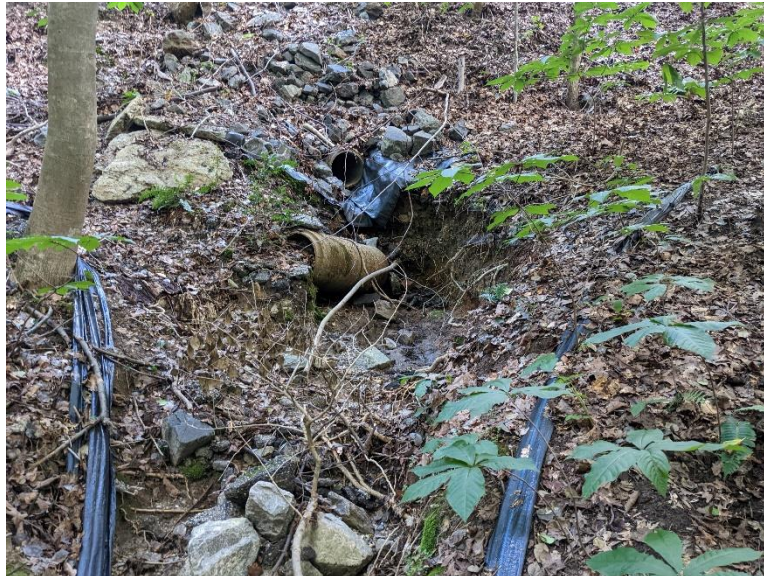
Site 1, Photo 1: Failed culvert near Horseshoe Drive (Looking Upstream (Northeast))
