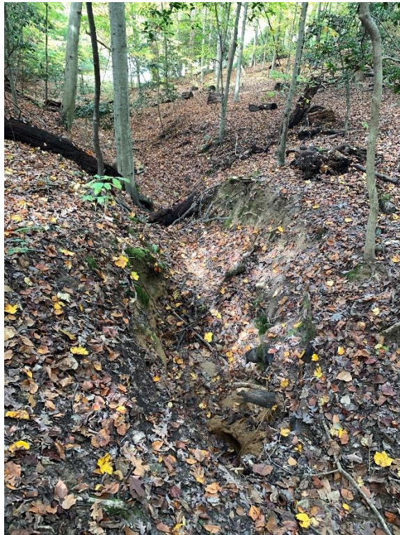
Site 1, Photo 6: Continuation of eroded ditch (Looking Downstream (West))
