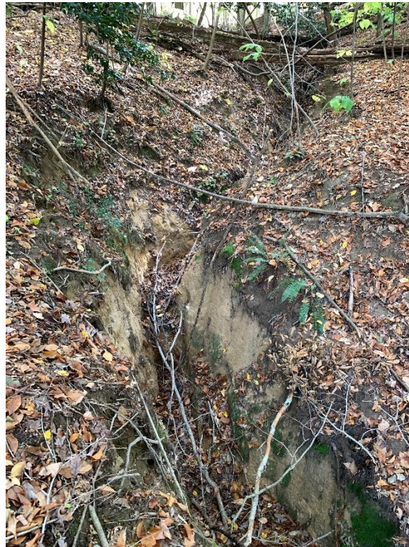
Site 5, Photo 7: Bottom of Eroded Ditch towards 271 Princess Place (Looking Upstream (Southeast))
