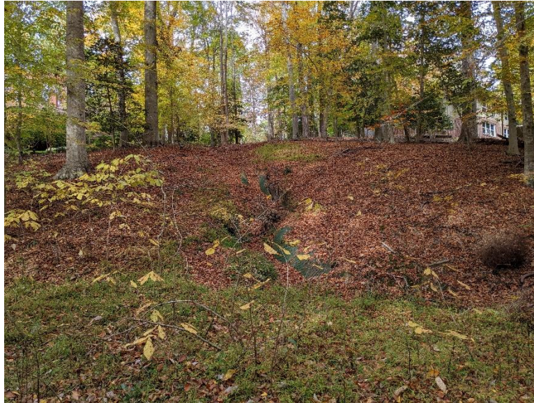
Site 4, Photo 13: Existing Geotextile Lined Channel at 104 Montague Circle (Bottom of Slope, Looking North)
