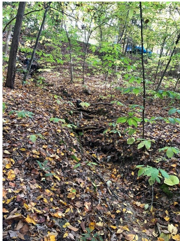
Site 1, Photo 2: Area downstream of failed culvert (Looking Upstream (Northeast))
