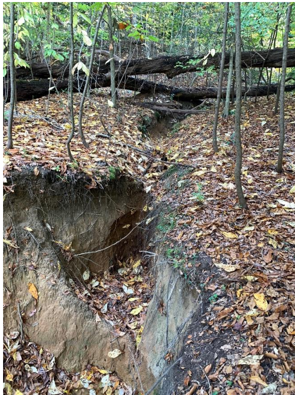
Site 8, Photo 6: Channel Erosion (Looking Upstream)
