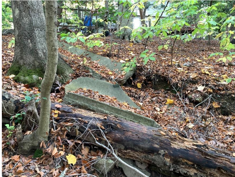
Site 6, Photo 7: End of Existing Damaged Concrete Channel at 103 North Will Scarlet Lane (Side View, Looking Northwest)
