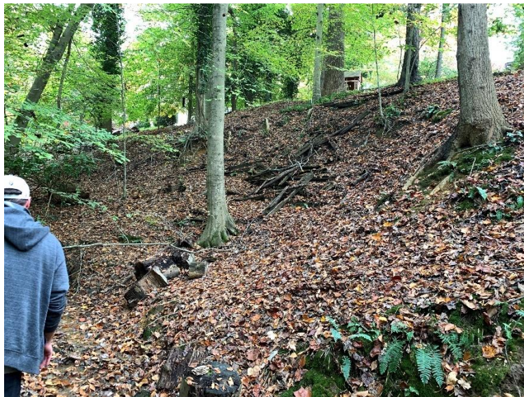
Site 3, Photo 4: Slope Erosion behind 260 Nottingham Road (Looking Southwest)
