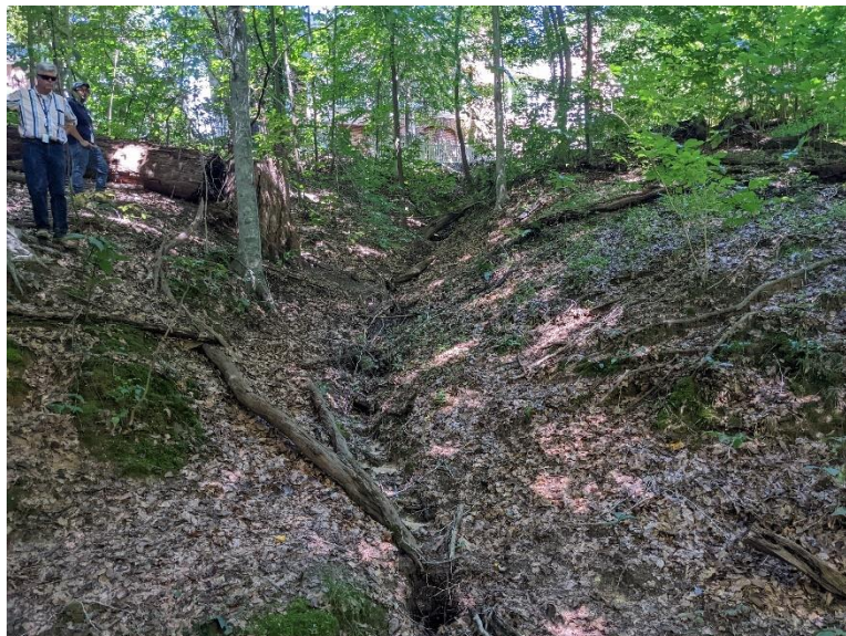
Site 4, Photo 6: Slope Erosion behind 266 East Queens Drive (Bottom of Slope, Looking North)
