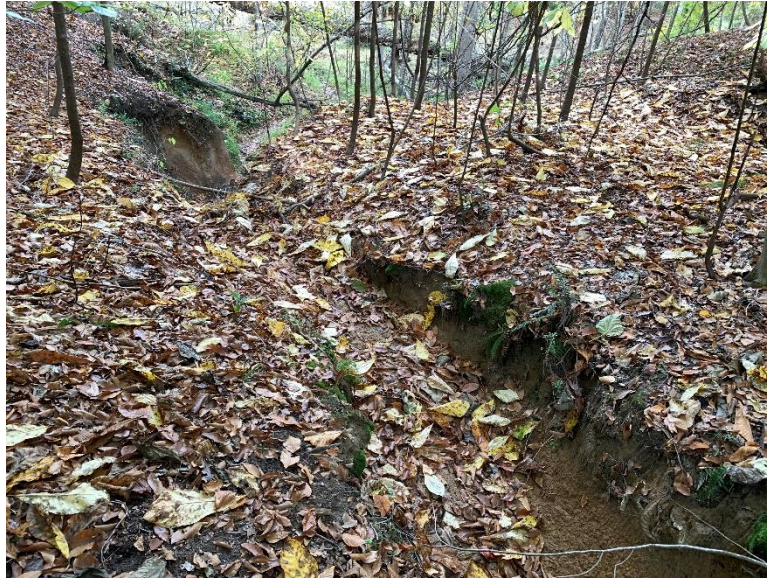
Site 8, Photo 5: Channel Erosion (Looking Downstream)
