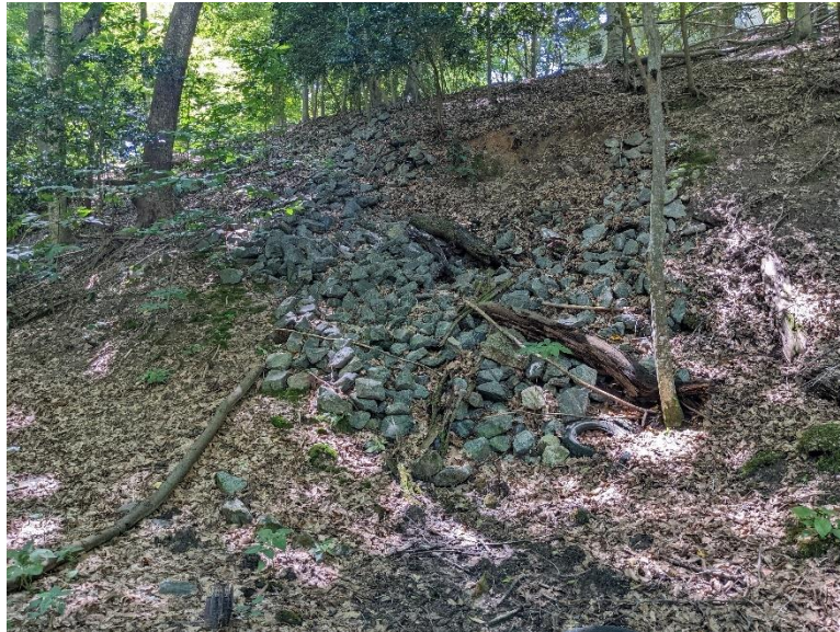
Site 6, Photo 2: Existing Rip Rap Slope Stabilization (Bottom of Slope, Looking Southwest)
