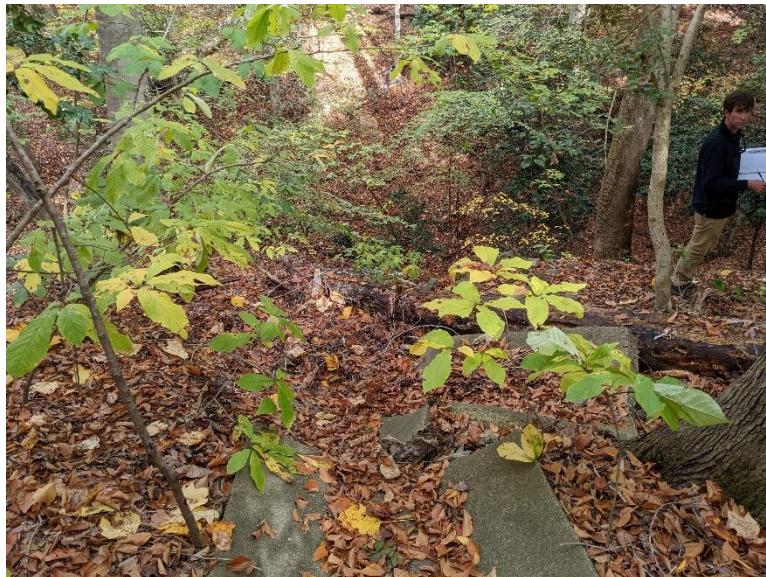
Site 6, Photo 6: End of Existing Damaged Concrete Channel at 103 North Will Scarlet Lane (Looking Downstream (Northeast))
