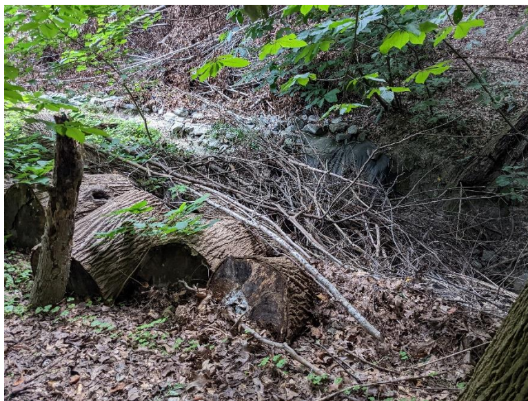
Site 2, Photo 4: Erosion at End of Existing Rip Rap (Looking Upstream (Northeast))
