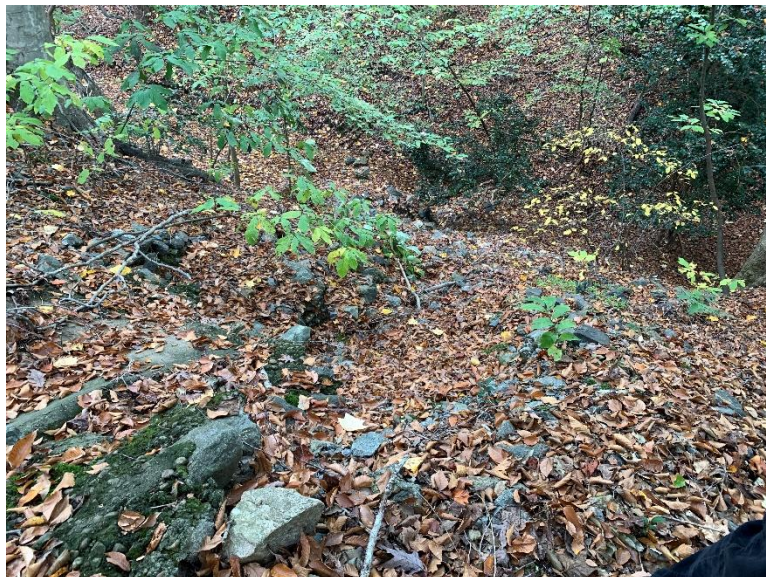
Site 6, Photo 8: End of Existing Concrete Channel / Existing Rip Rap Slope Stabilization (Top of Slope, Looking Northeast)
