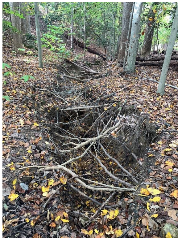
Site 1, Photo 4: Eroded ditch downstream of failed culvert (Looking Downstream (West))
