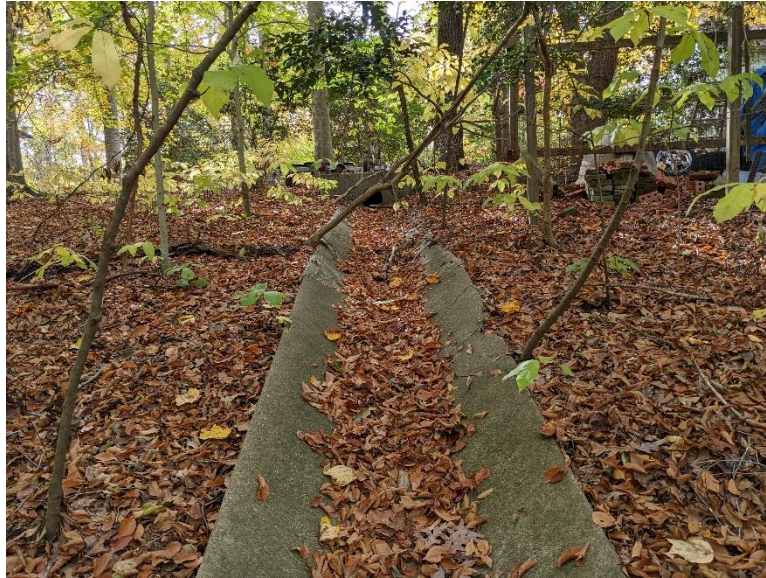
Site 6, Photo 5: Existing Concrete Channel at 103 North Will Scarlet Lane (Looking Upstream (Southwest))
