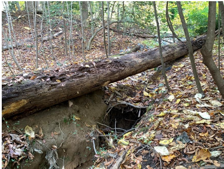
Site 8, Photo 4: Beginning of Channel Erosion (Looking Upstream)
