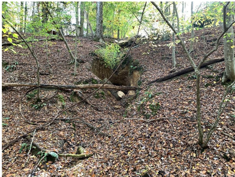
Site 4, Photo 14: Severe Erosion between 104 and 106 Crown Court (Bottom of Slope, Looking South)
